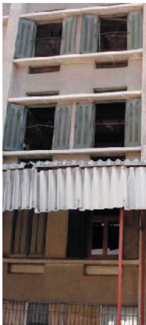
Building used for cocoon storage above and offices for cocoon producers association below.
